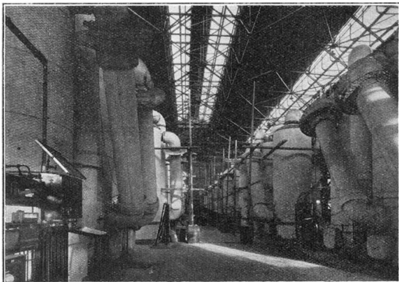
FIG. 2.—New hydrogen plant.
