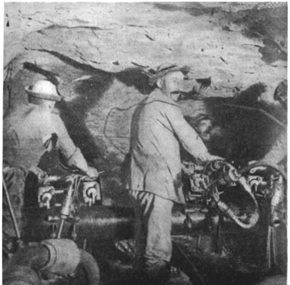
FIG. 2.—The Brandt drill at work at the "face." Daily progress 18 feet. Size of heading 10 feet x 6 feet.
