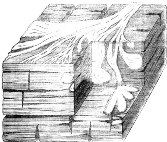
FIG. 13.—A piece of pine-wood attacked by the mycelium of Polyporus vaporarius . The timber has warped and cracked under the action of the fungus, becoming of a warm brown colour at the same time; in the crevices the white strands of felt-like mycelium have then increased, and on splitting the diseased timber they are found creeping and applying themselves to all the surfaces. Except that the colour is snowy white, instead of gray, this mycelium may easily be mistaken for that of Merulius . The fructification which it develops is, however, very different. (After R. Hartig.)
