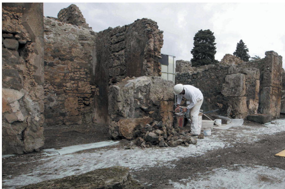
Conservation work under the Great Pompeii Project began at the site in 2013.
