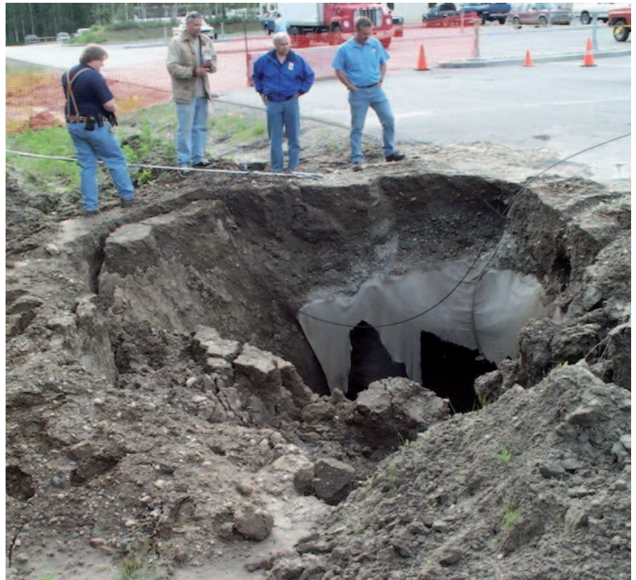
Collapse caused by thawing permafrost at the edge of the Geophysical Institute parking lot at the University of Alaska, Fairbanks.
