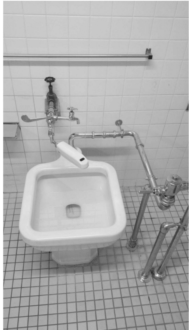
Figure 5 A picture of automatic flushing toilet for disposing of urine or waste without touching a lever.
