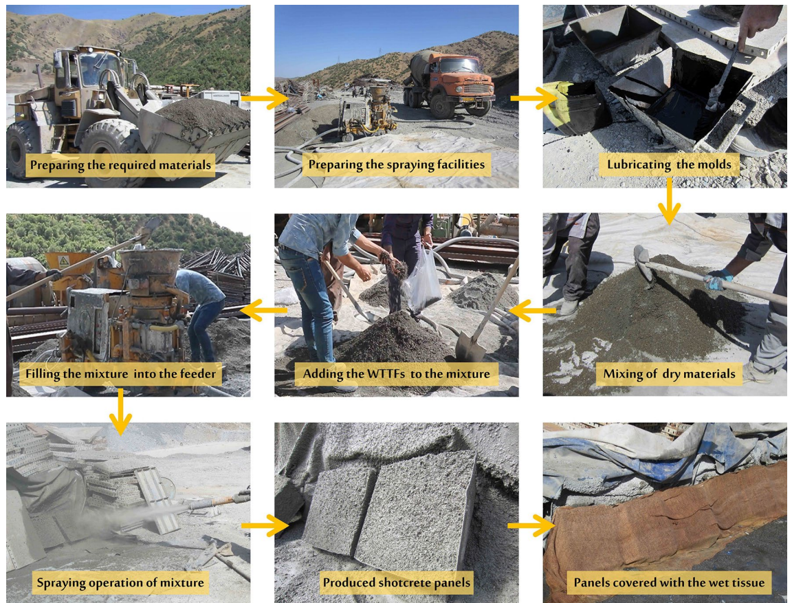
Figure 4. Shotcrete specimen production operations at the site of the Bagan–Mariwan Tunnel project.
