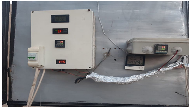
Figure 4. Image of control units.
