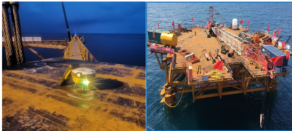
Figure 12. Platform top monitoring instrument and platform accurate installation diagram (photographs are derived from the project works by the author of this article).
