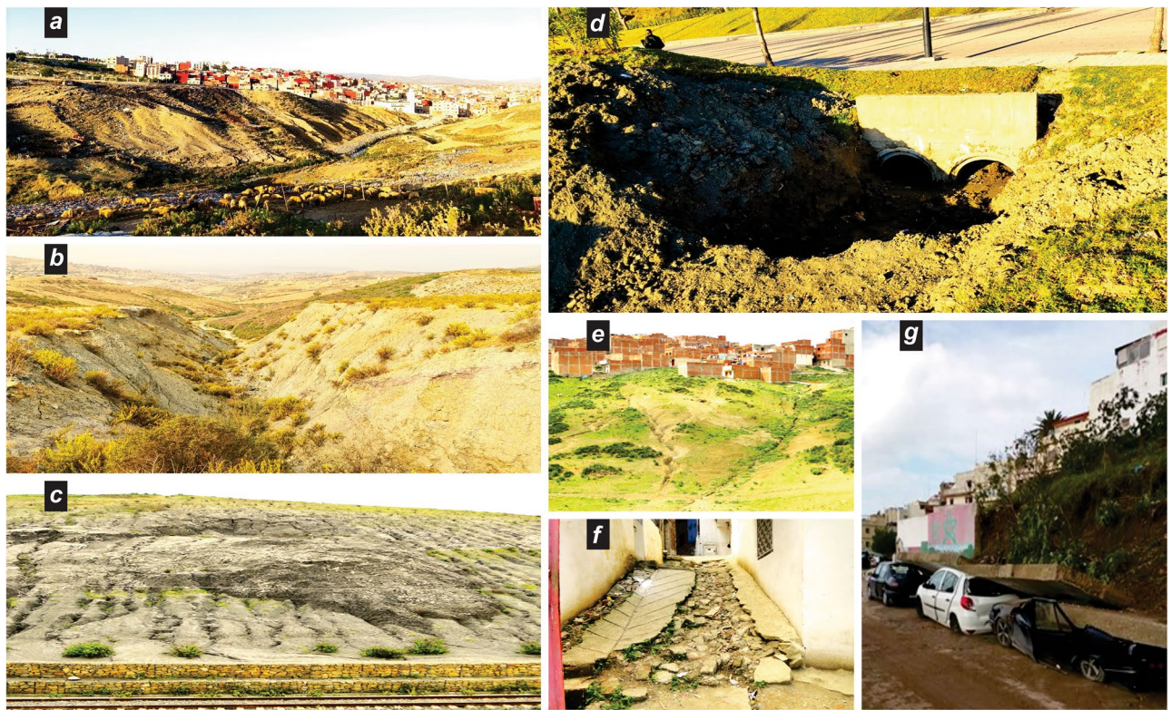
Figure 6. Inadequate upstream measures leading to drainage channel blockages and examples of consequent damage. (a) Muds and debris clogging drainage in a waterway in an outlying neighborhood; (b) erosion canyon overlooking hydrographic axis flowing towards industrial zone and Mghougha depression flood barrier; (c) mass landslide upstream of the Mghougha sub-basin; (d) complete obstruction of essential drainage channels; (e) evolution of erosion shapes in the vicinity of upstream semi-urban areas; (f) damage to alleyways and public walkways turned into natural drainage channels for torrents; (g) damage to properties resulting from land degradation. Credits attribution: pictures from the authors.
