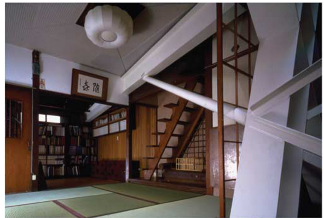
Figure 3 | The new steel frame is clearly distinguished from the old timber structure. © Katsuhiro Miyamoto. This image is reproduced with permission of the copyright holder, and is not covered by a Creative Commons Attribution 4.0 International License.
