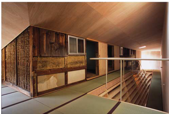
Figure 7 | The interior space where the old house is stabilised by the new insertion. © Katsuhiko Miyamoto. This image is reproduced with permission of the copyright holder, and is not covered by a Creative Commons Attribution 4.0 International License.
