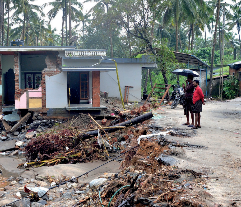
Houses destroyed by a landslide in Kerala, India, after exceptionally heavy rain in August.
