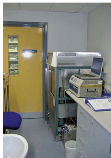
Fig. 3 Sterilisation section of three part decontamination unit
