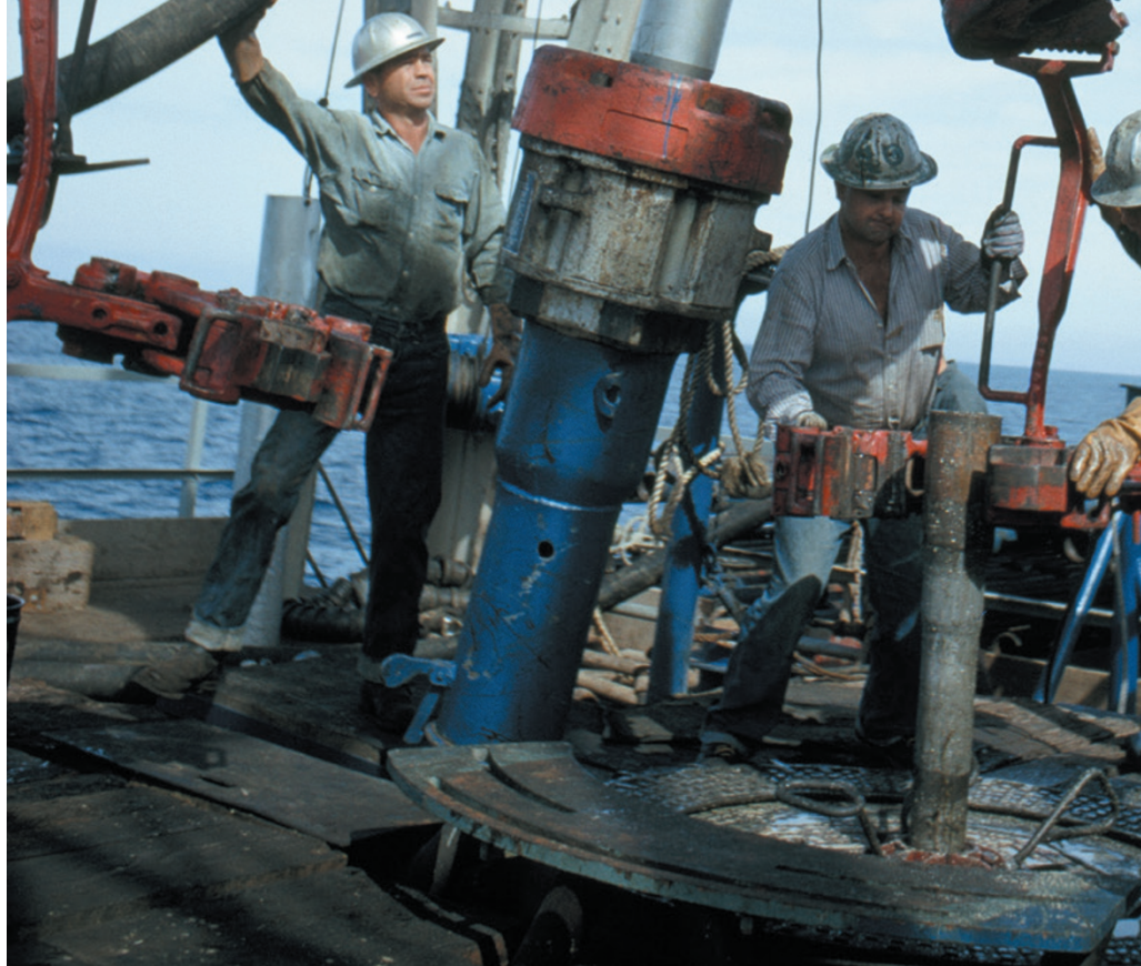
Crews lower huge drills down from specially equipped ships to penetrate the sea floor.
