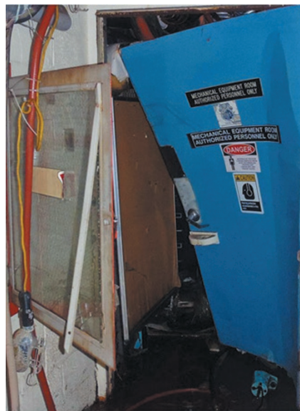
A steel door pushed in by Hurricane Sandy at the NYU Langone Medical Center.
