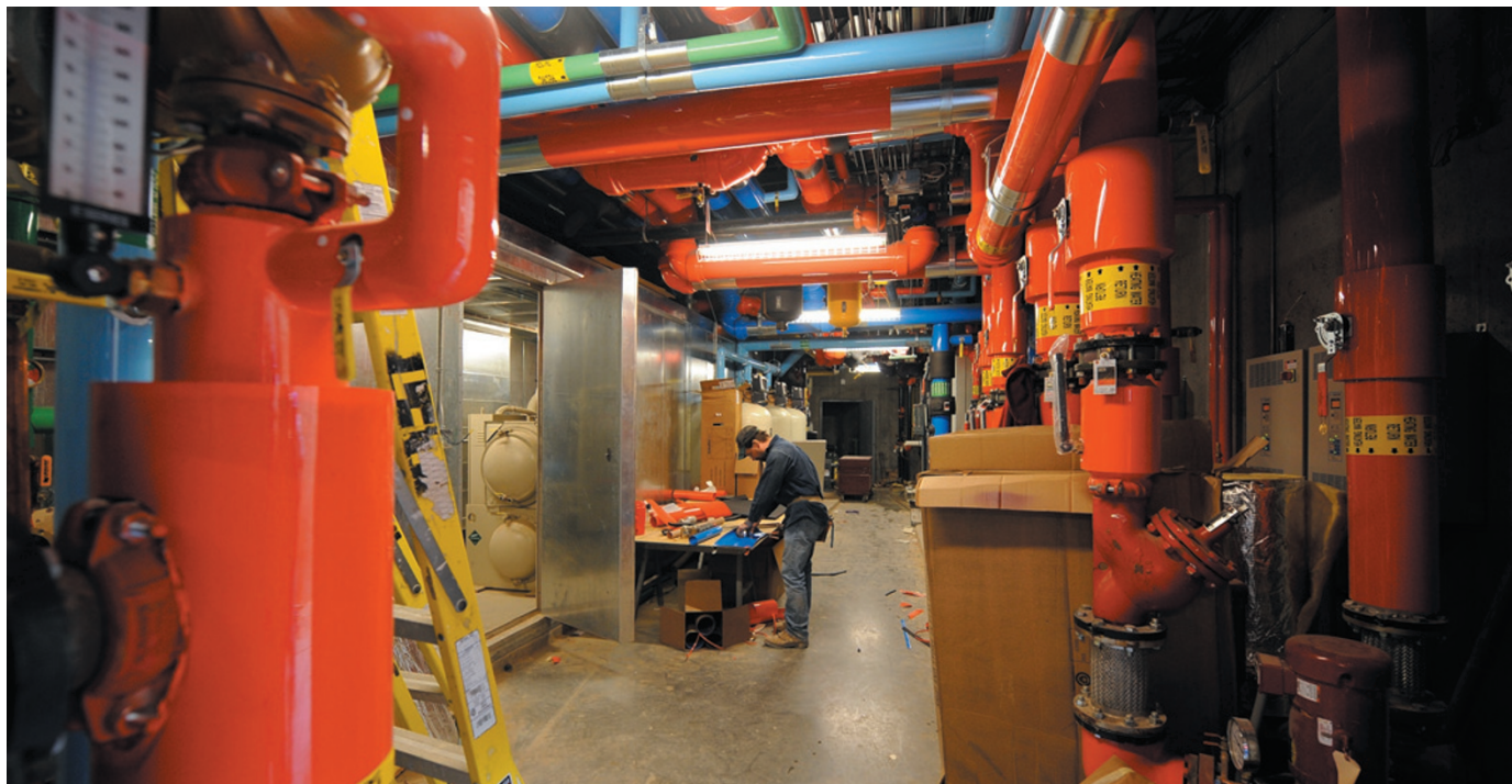
A heating and cooling system based on geothermal energy at a hospital in Greensburg, Kansas.
