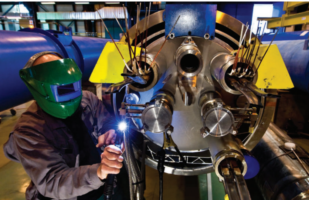
It took months to repair magnets that were damaged in a major accident to the LHC in September 2008.
