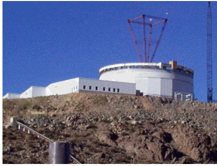
Going up: the Gemini facility at Cerro Pachon, Chile, pictured last month.
