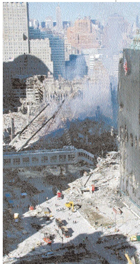
Devastation: workers remove rubble after the collapse of the World Trade Center.
