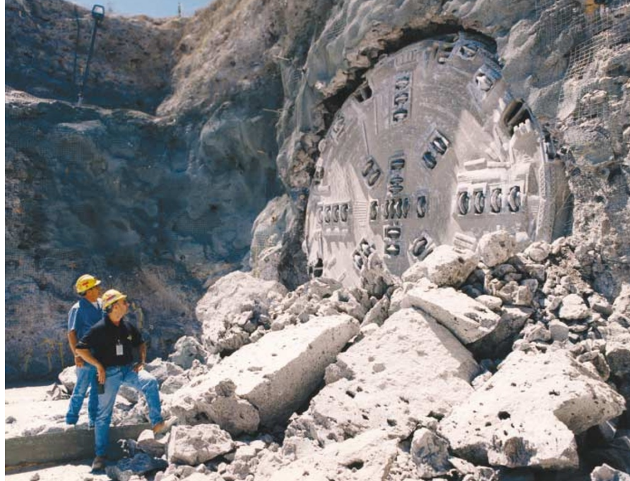
Digging that scene: project engineers watch the completion of the main test tunnel at Yucca Mountain.
