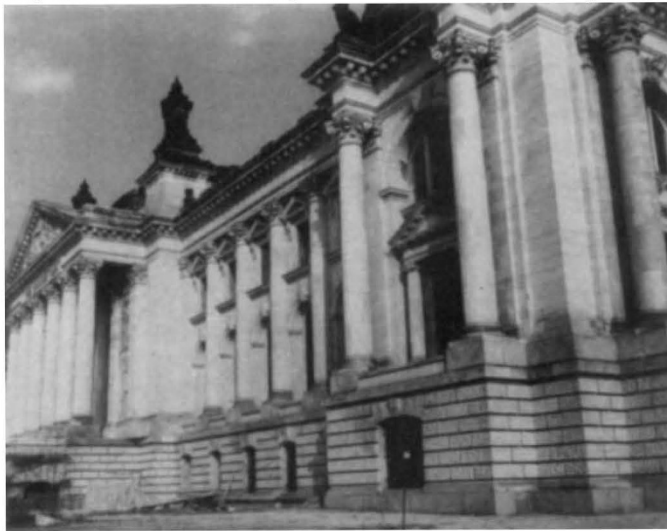
Work is progressing on the reconstruction of the Reichstag building, gutted by fire in 1933 at the time the Nazis rose to power and wiped out parliamentary democracy in Germany.
