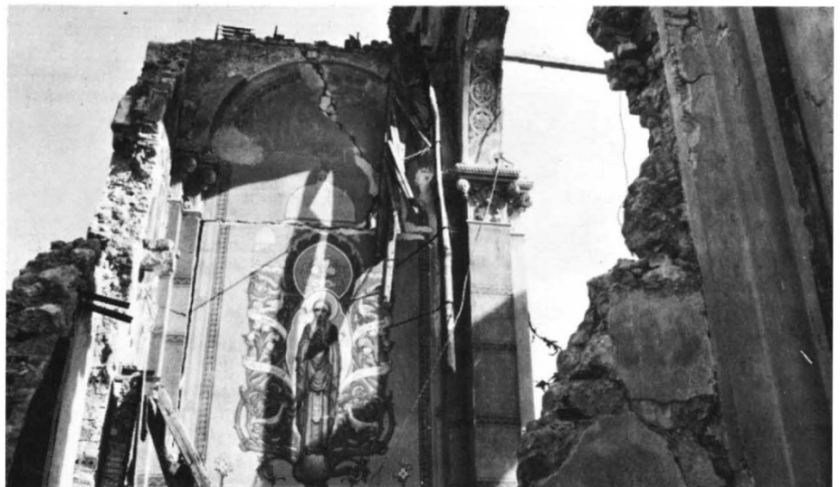
Destruction at Friuli
