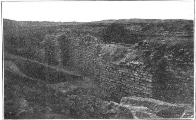
FIG. 1.—Part of the buttressed outer wall of E-nun-makh, the temple of the Moon-god and his consort. The lower part was built by Bur-Sin (2250 B.C.), the upper part by Kudur-Mabug (2000 B.C.); the interior brickwork seen above is by Nabonidus, last king of Babylon (c. 550 B.C.). By courtesy of the trustees of the British Museum and the Board of the University Museum, Philadelphia.
